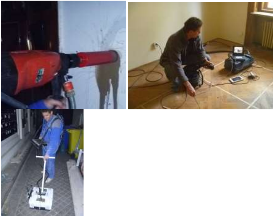
Figure 12. Diagnostic assessment of the building, from left to right: core drilling, videoendoscopy, radar survey.
