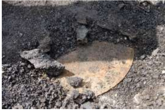
Figure 8. Sinkhole covered with metal plate under the pavement layers.
